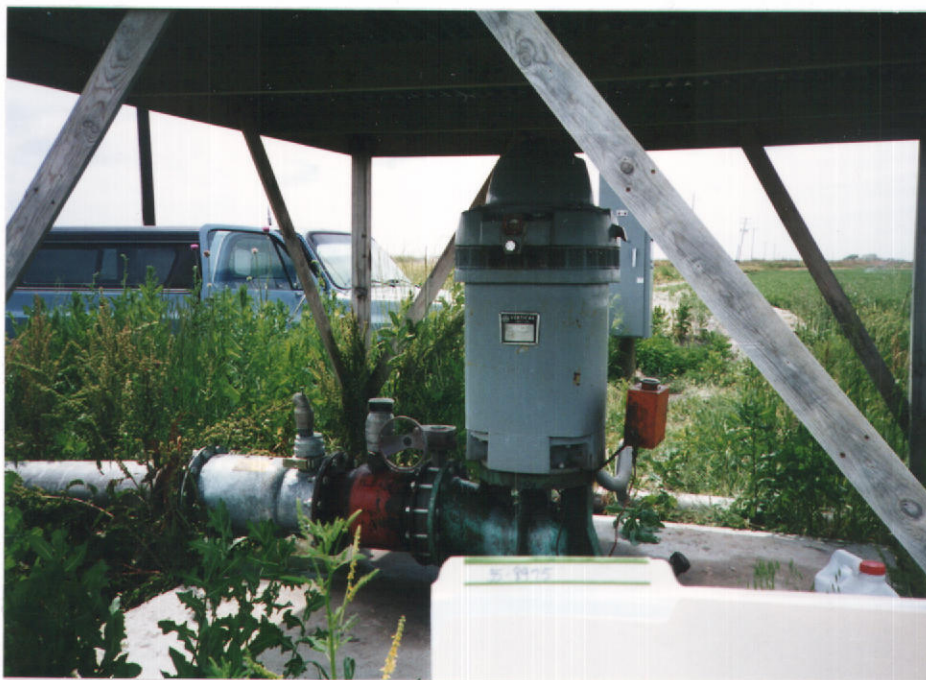
Plate 1 - Motor and pump assembly at point of diversion.
