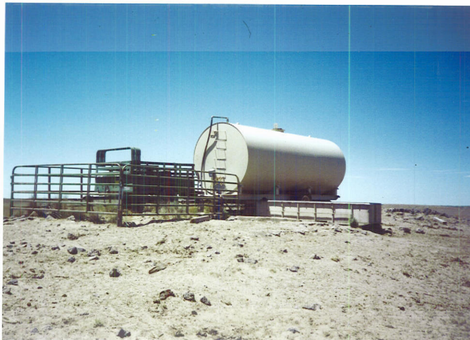
Fig. 2 - Complete system showing 1000 gallon storage tank, stockwater trough and generator.
