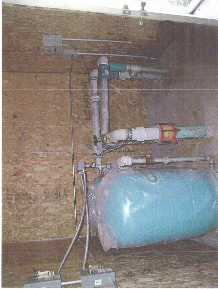
35-9058 well house / pressure tanks.
