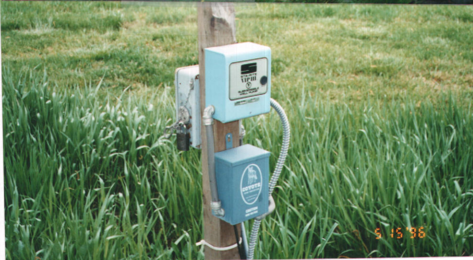
power box for pump
