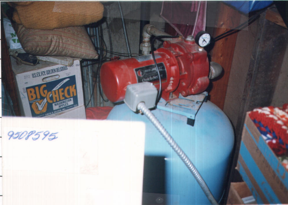
PRESSURE Pump & TANK
