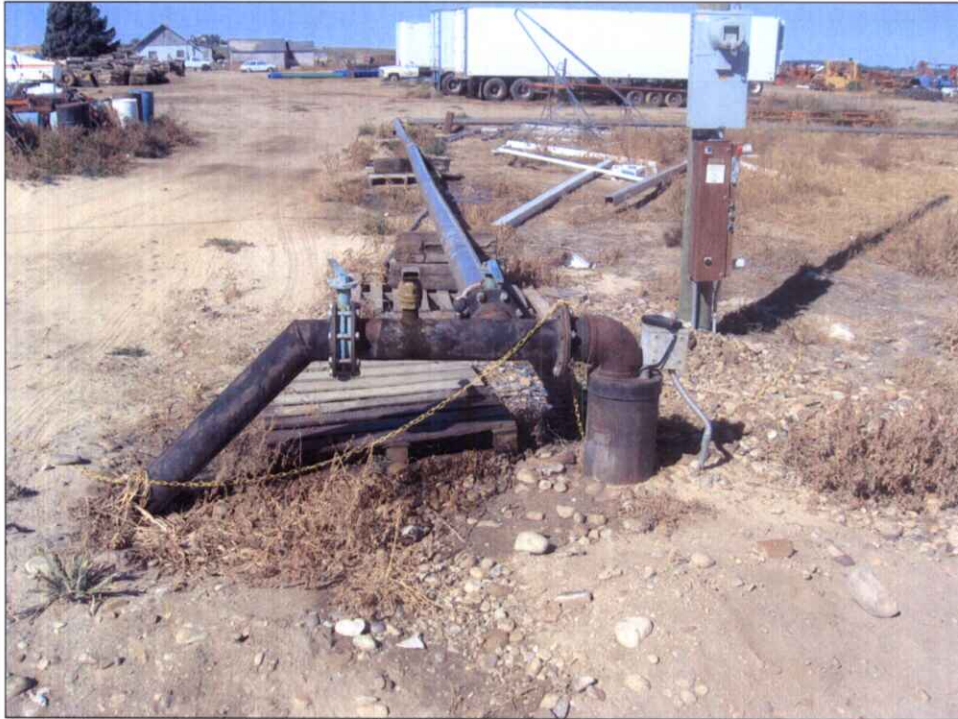
Photo 1: Taken at point of diversion facing west. Southern (left) butterfly valve is closed; northern butterfly valve is open.
