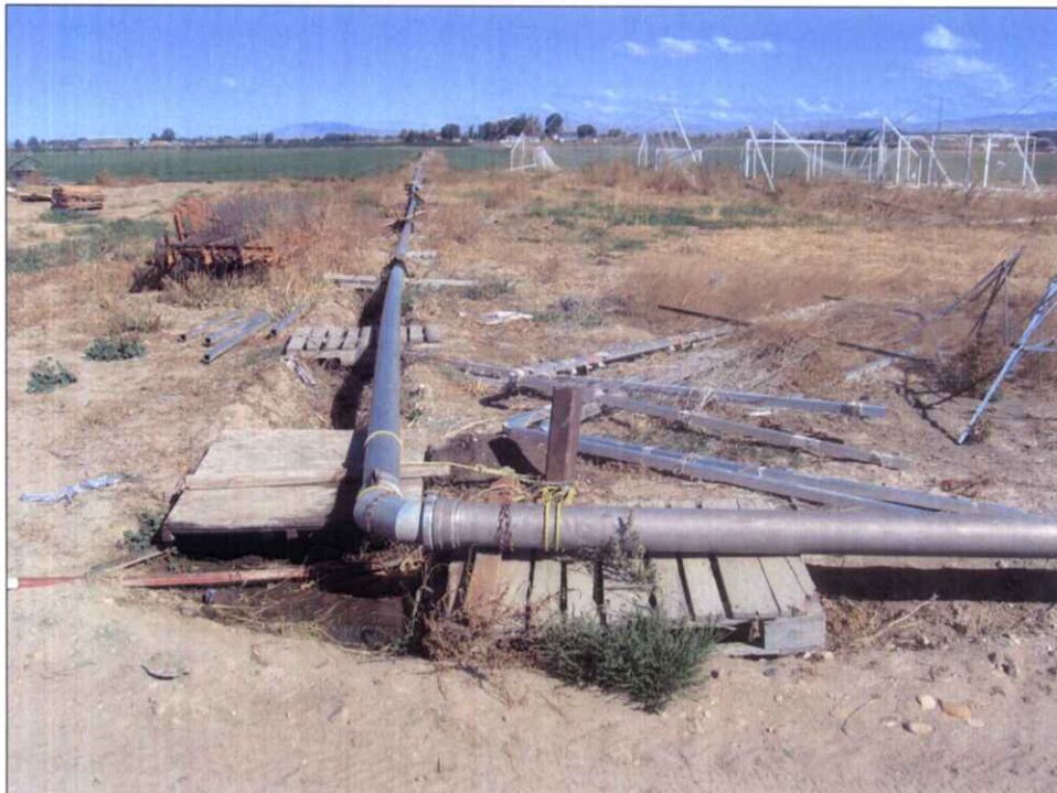
Photo 2: Taken 40-feet west of well, facing north. Well is to the right; place of use is right (east) of 6-inch aluminum mainline.
