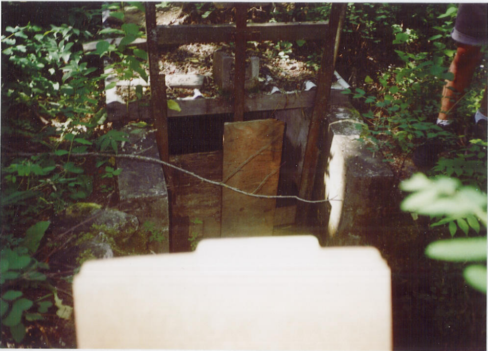
P.D. ← Control Box on SAGE Creek
