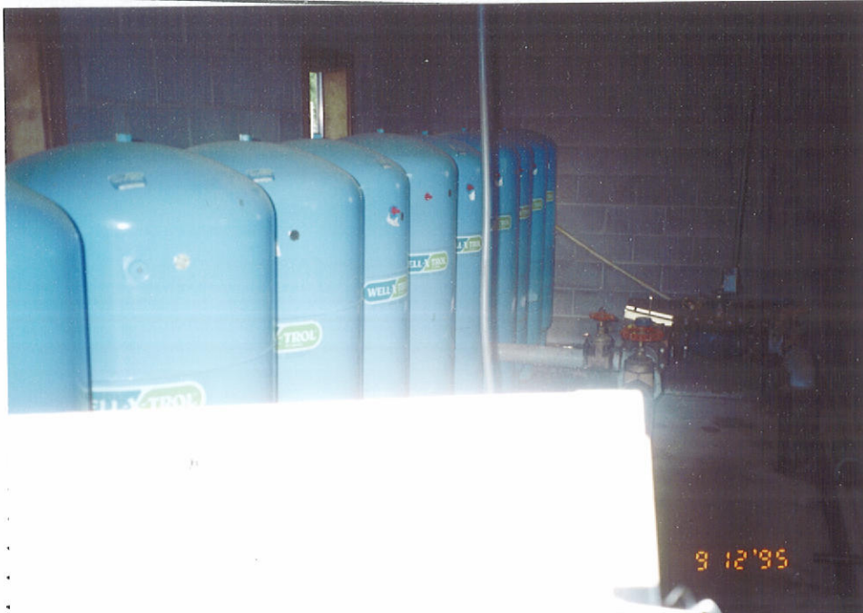
PUMP PRESSURE TANKS
