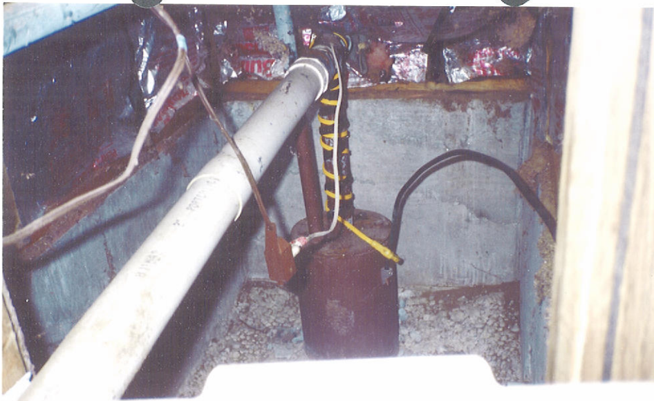
P.D. Pump To Storage WELL CASING
