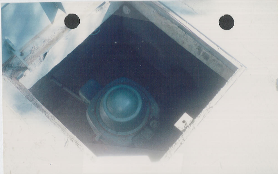
Pump AT GROUSE CREEK
