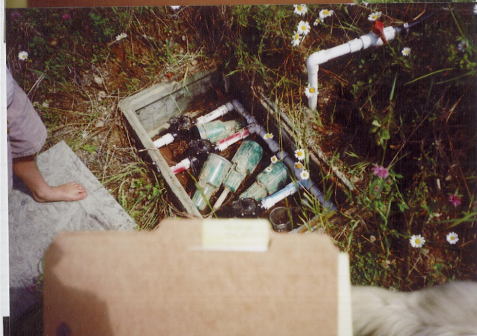
← SPRINKLER HEADS AND SPLIT
