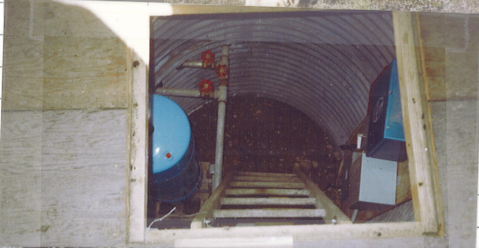
INSIDE PUMP HOUSE
