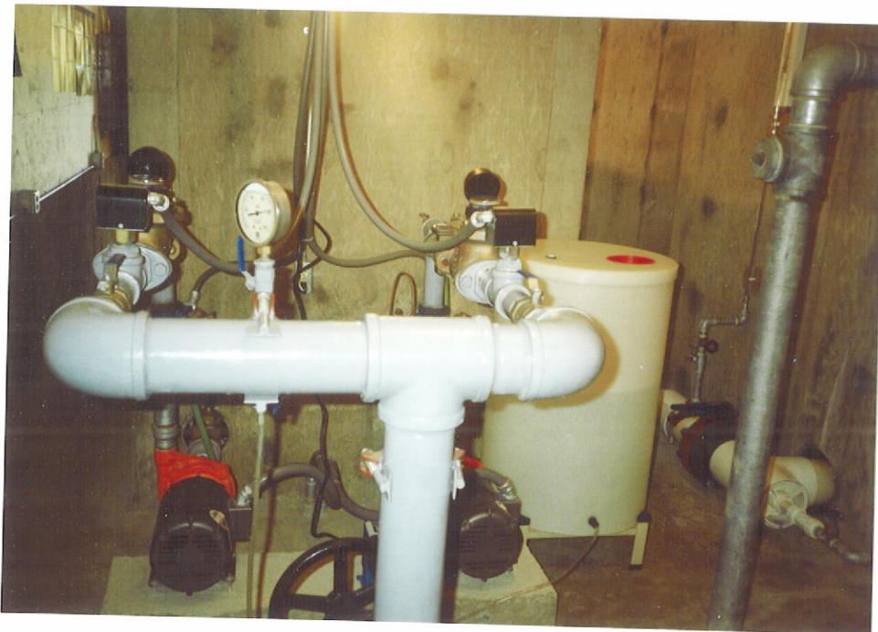
Clear Well & Booster Pumps
