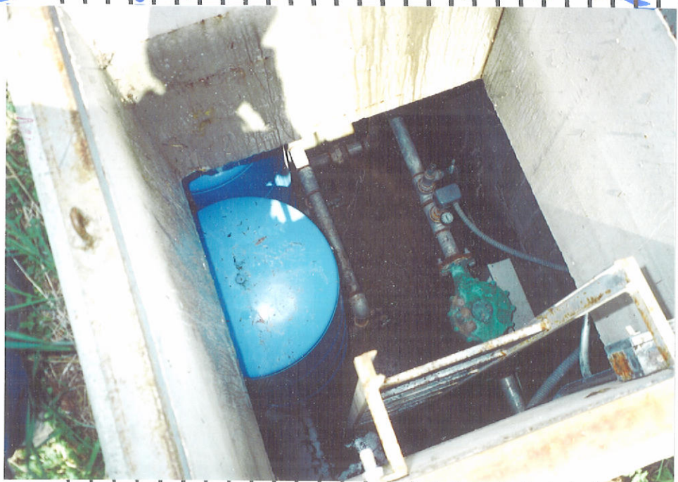
Flow meter - Looking in Concrete Bunker
