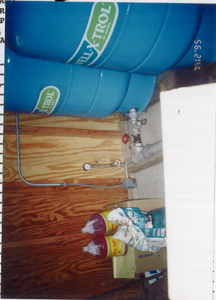
7.5 HP PUMP 3 PRESSURE TANKS
