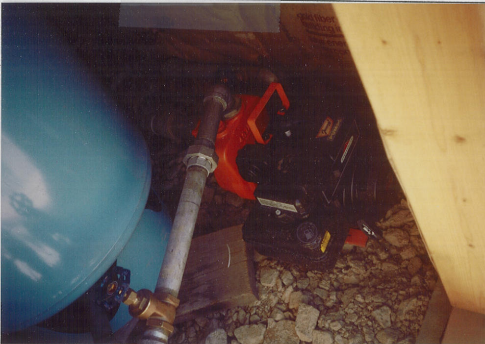
Back-up "fire" pump
