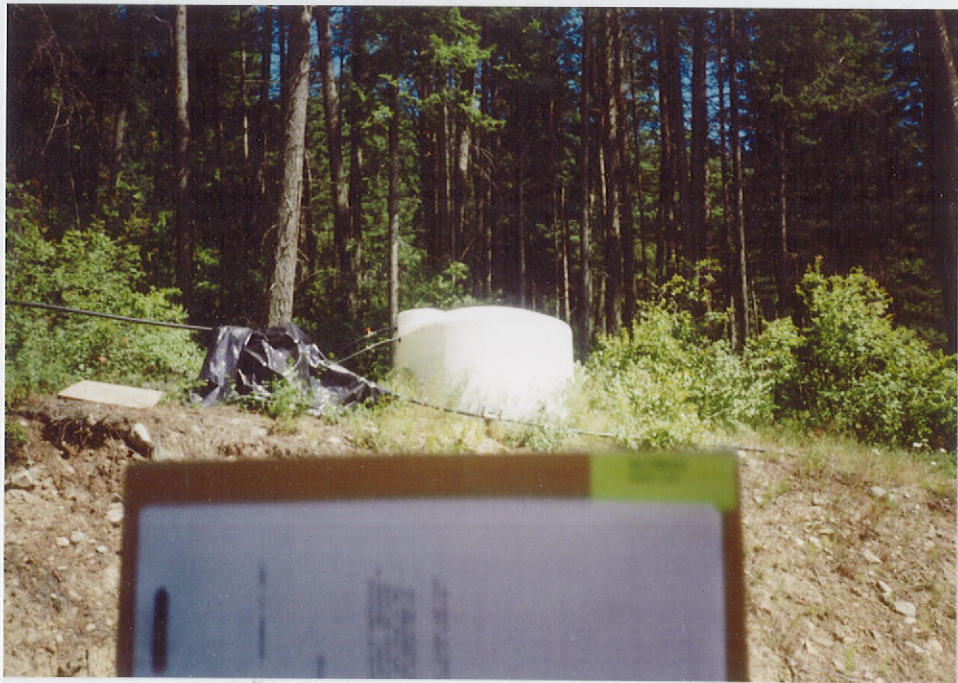
1550 gall ← STORAGE TANK
