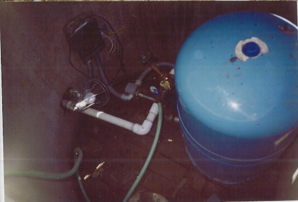
Delivery system w/ 40 gallon hold 45 PSI
