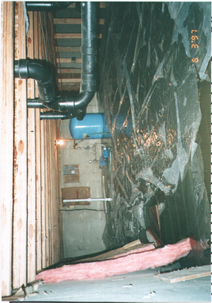
Pump and Pressure Tank
