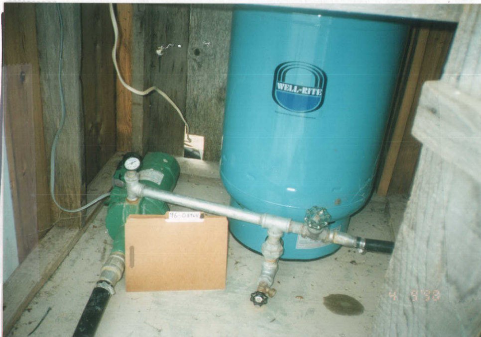
Pump / Pressure tank
