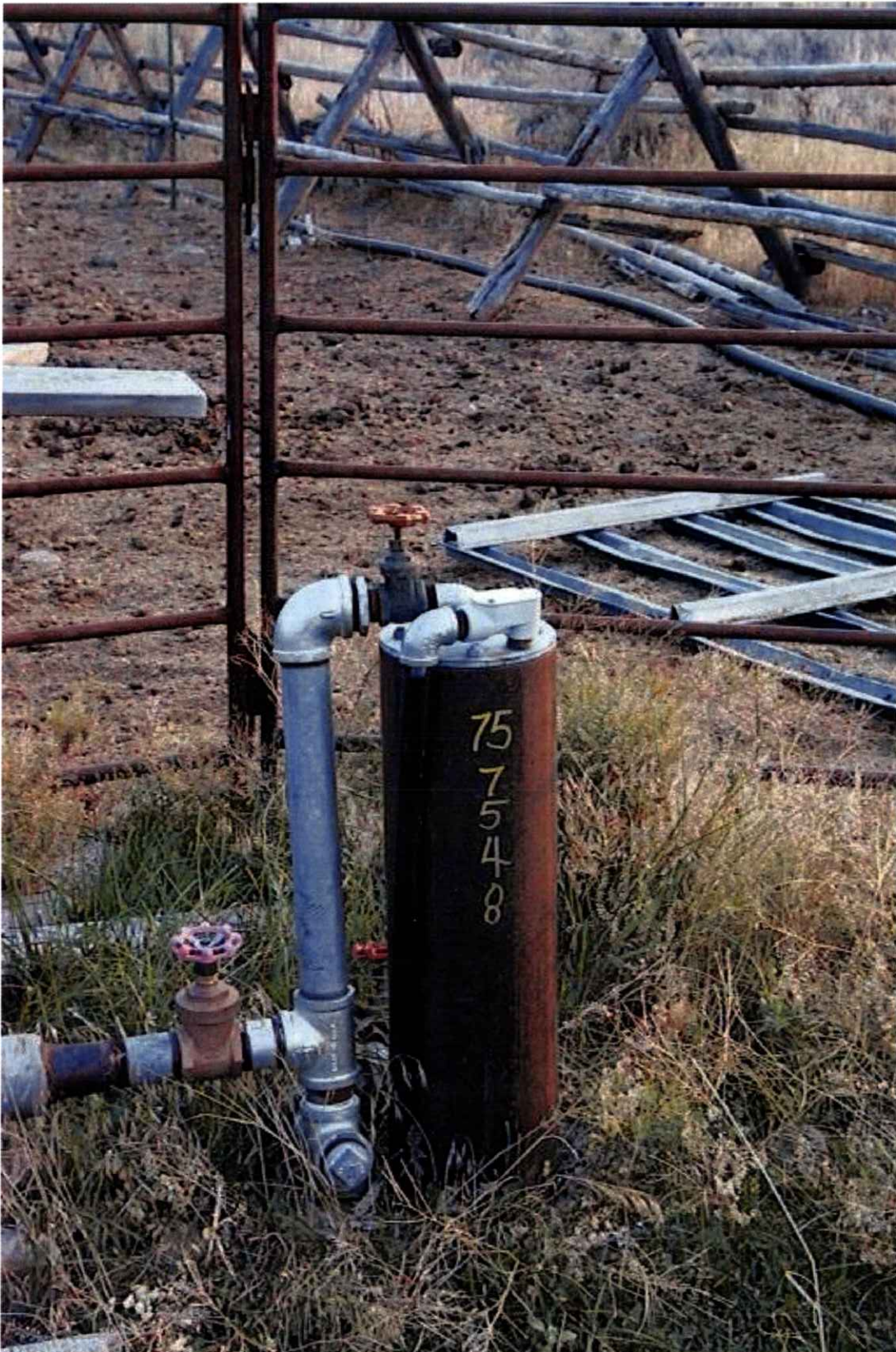
View #2 P/D with black PVC Mainline under fence.
