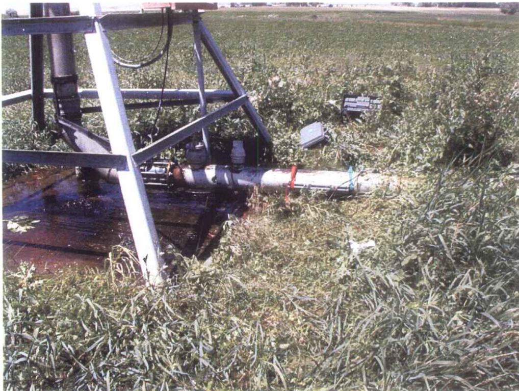
South pivot flow measurement
