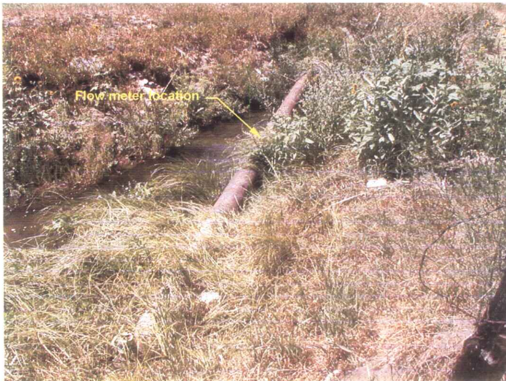
HL1 mainline flow measurement
