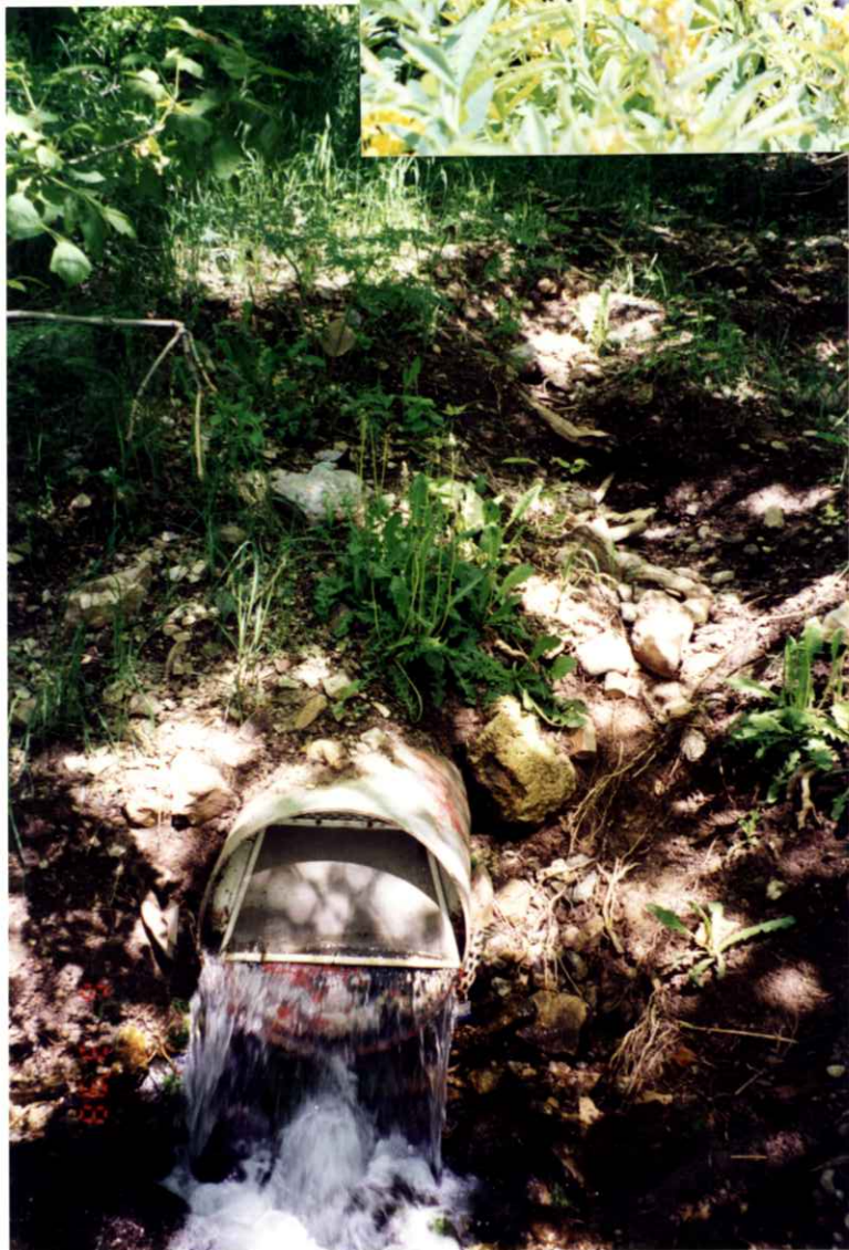
STORAGE TANK OVER FLOW ←
