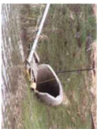
outlet for large pond and POD outlet
