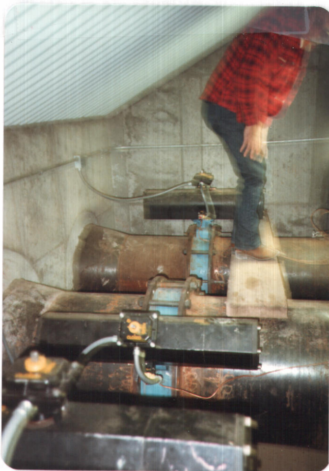
Bottlet/1 Control Valves on Turbine inlets
