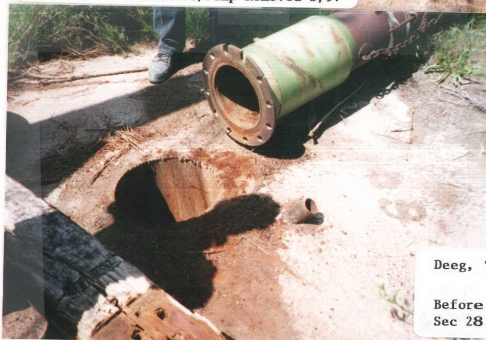
Well to be Abandoned/Pump Removed 5/97
