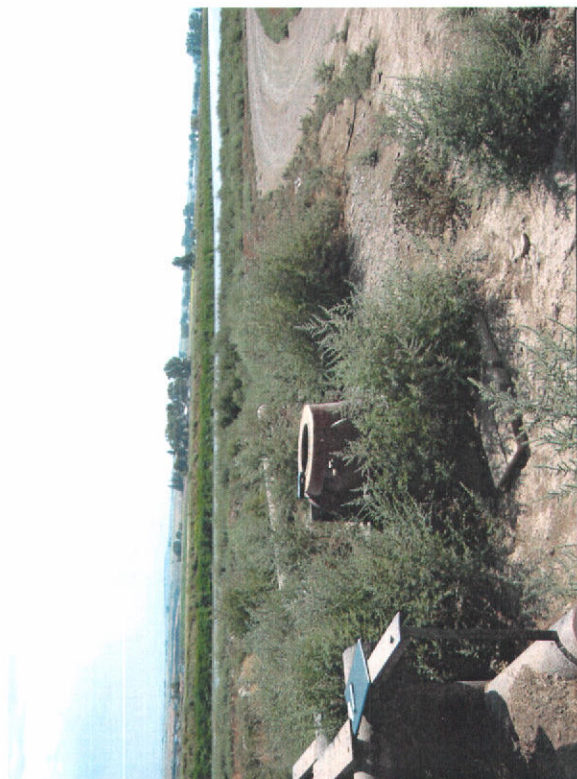
Photo taken September 5, 2002. Well located in the SWNWSE Section 36. Re-bored and pump tested summer 2002. Permittee in process of bringing power into site.
