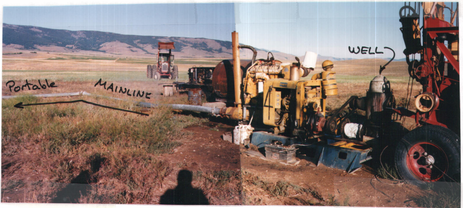
SOUTH VIEW OF WELL, PUMP & MOTOR
