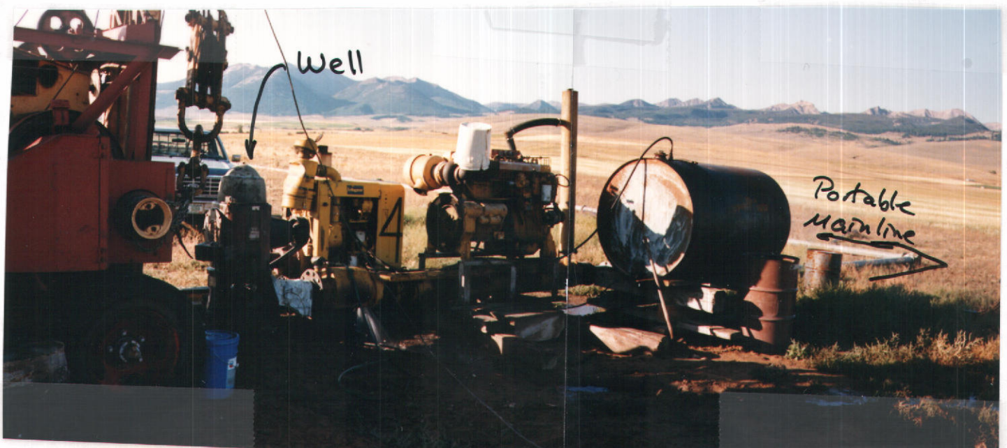
NORTH VIEW WELL PUMP & Motor
