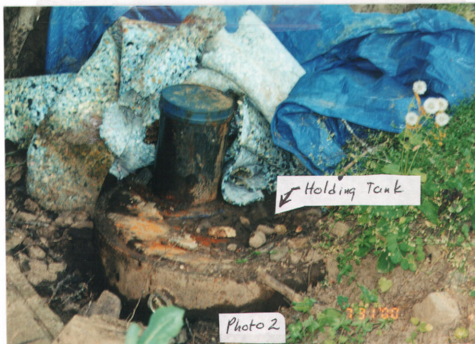
Photo 2. Showing holding tank and well head.
