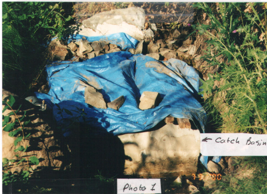
Photo 1. Showing catch basin in spring.
