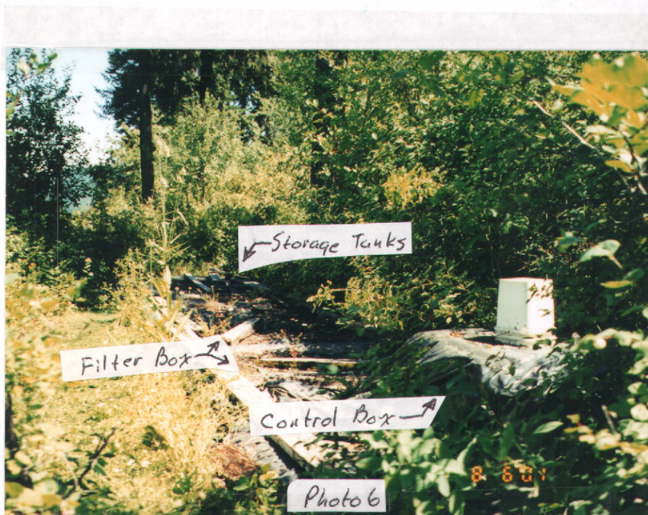
Photo 6. Showing configuration of control box, filter box, and storage tanks.
