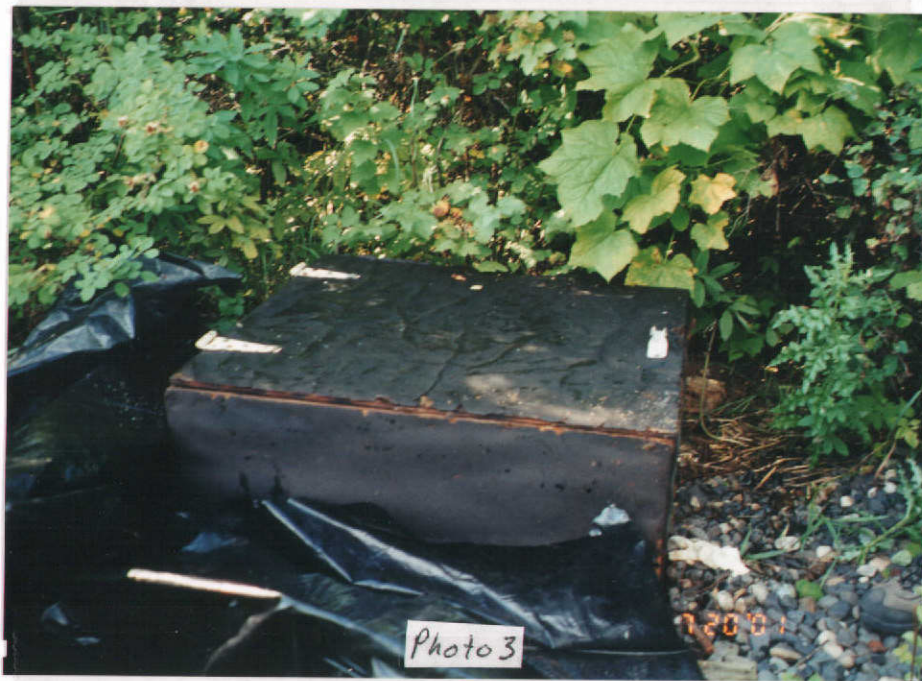
Photo 3. Showing outside of control box.
