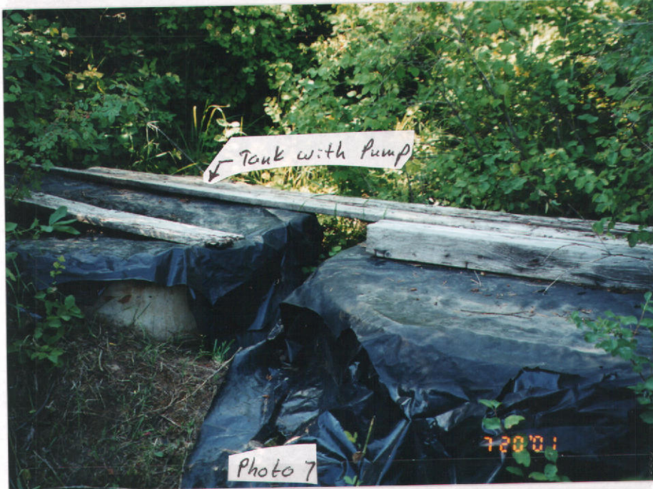
Photo 7. Showing the two storage tanks.
