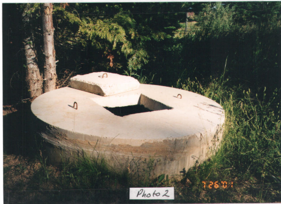
Photo 2. Showing storage tank.
