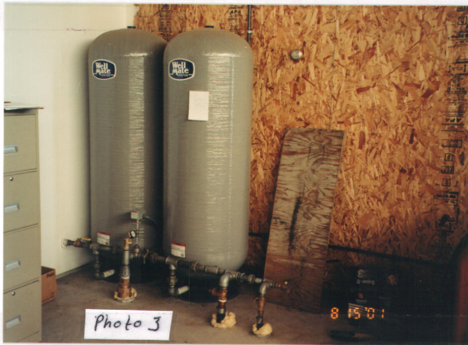
Photo 3. Showing pressure tanks in shop.
