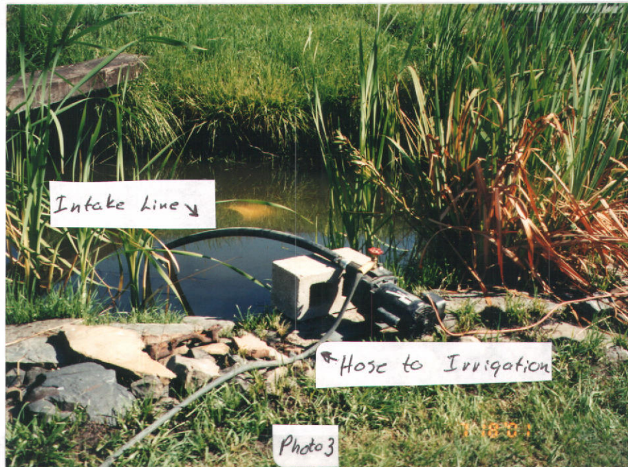
Photo 3. Showing irrigation pump.
