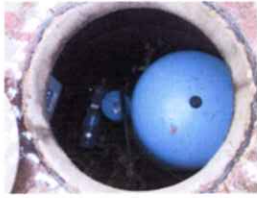
PUMP AND PRESSURE TANK
