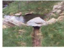
PIPE FROM LARGE POND TO SMALL POND 2
