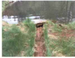
PIPE FROM LARGE POND TO SMALL POND
