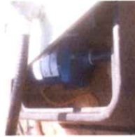
PUMP AT SPRING
