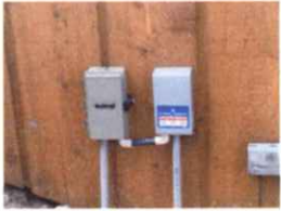
CONTROLS FOR LAWN IRRIGATION SYSTEM
