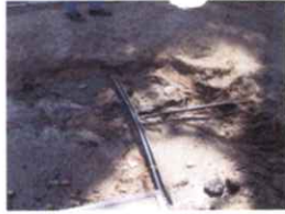
PIPES COMING OUT OF THE LAKE
