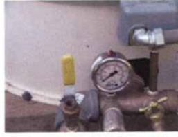
CURRENT PRESSURE OF SYSTEM
