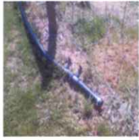
IRRIGATION LINE WITH HOSE CONNECTIONS.jpg
