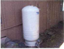
PRESSURE TANK FOR WATER SYSTEM
