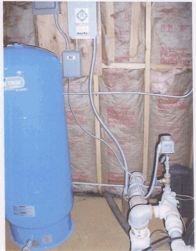
Figure 2: Point of Diversion (Well #2) for Southern Comfort HOA.
