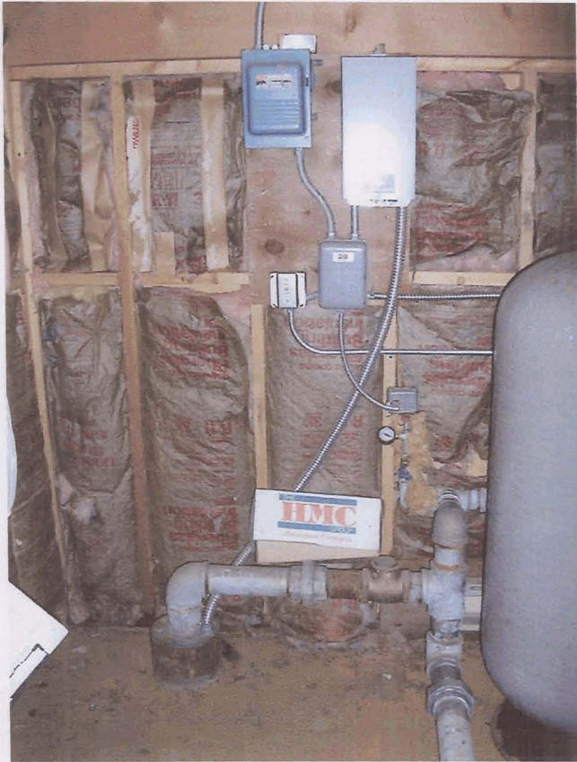
Figure 1: Point of Diversion (Well #1) for Southern Comfort HOA.
