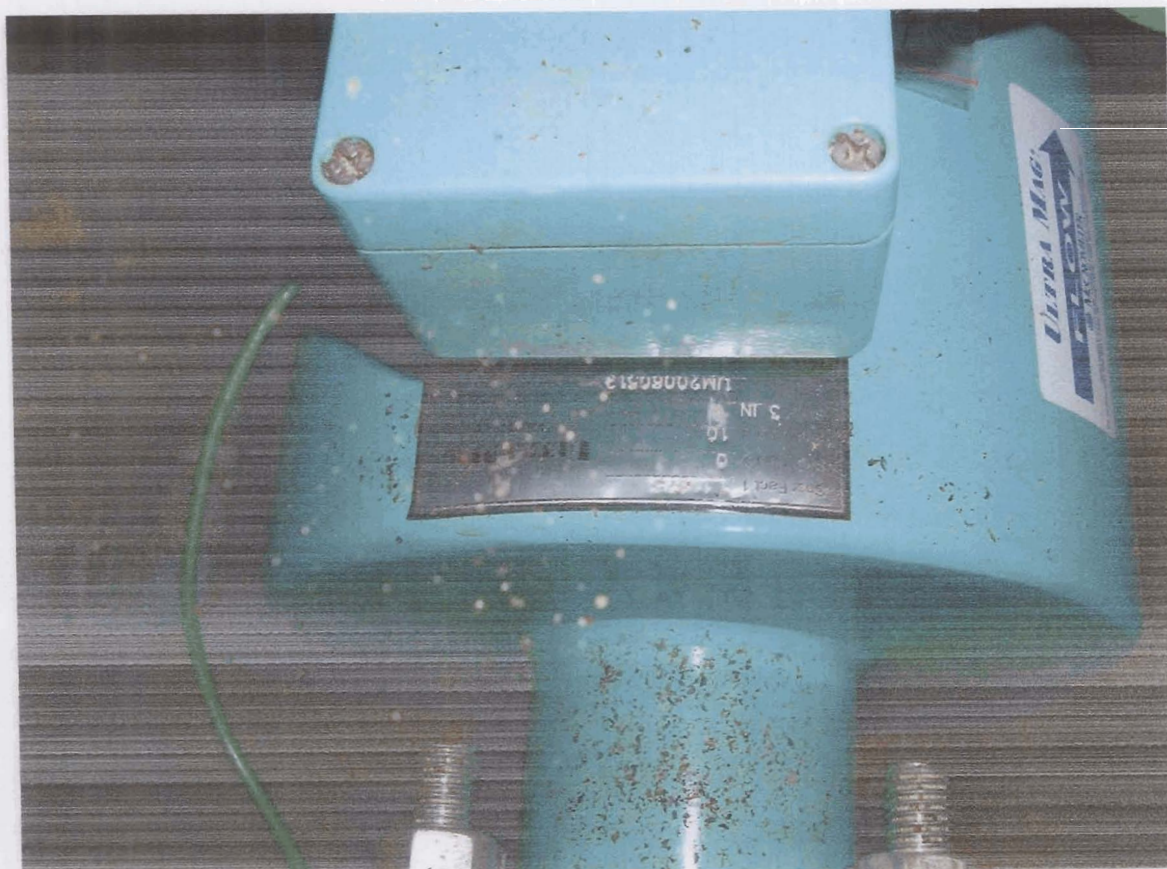
Figure 5: McCrometer UltraMag Flow meter for Well #2.
