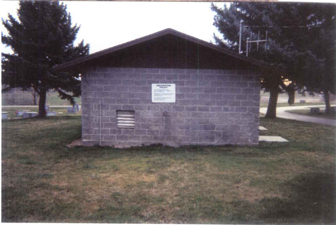
Figure 5. Photographs of the Caldwell Well #4-B pump control house. The upper view shows the Well #4-B in the foreground and looks west to the east wall of the control house with Canyon Hill Cemetery in the background. The lower view is of the west side of the pump control house.
