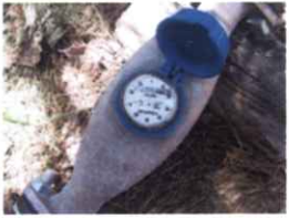
METER ON SYSTEM
