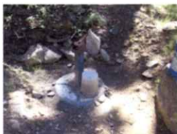
92-10023 well above valve station.JPG
