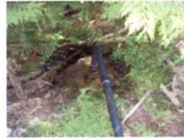
92-10023 Reservoir overflow back to stream.JPG
