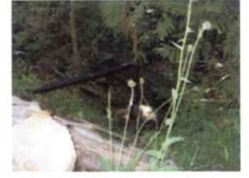
92-10023 Gravity fed pipe reservoir to house.JPG
