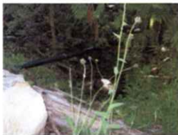
92-10023 Reservoir -Valve Station pipe.JPG
