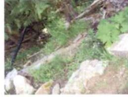
92-10023 Pipe from reservoir to house.JPG
