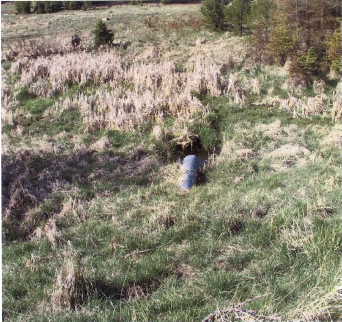
POINT OF DIVERSION OUTLET
