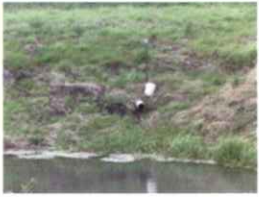
INLET FROM FIELD DRAINAGE
