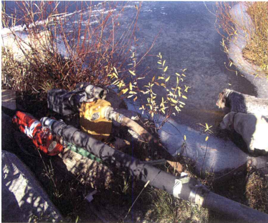
P/D: Red 2 hp pump and yellow 8 hp pump
