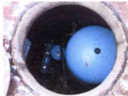
PUMP AND PRESSURE TANK
