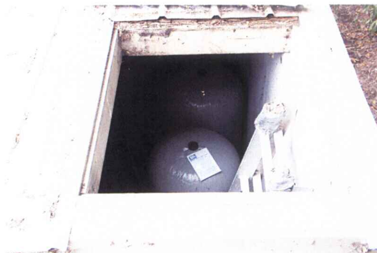
Underground storage of two pressure tanks. 1 for each home.
