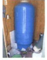
PRESSURE TANK AND SYSTEM
