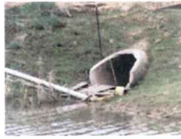
outlet for large pond and POD outlet
